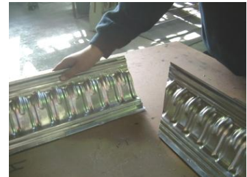
6/Picture shows left hand cornice still left "square" installing. Right hand cornice has been mitred.
