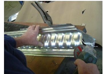
3/ Move along in Mitre Box approx. 100mm. Clamp to hold in place prior to cutting, cut 5mm to the outer side of scribed line.
